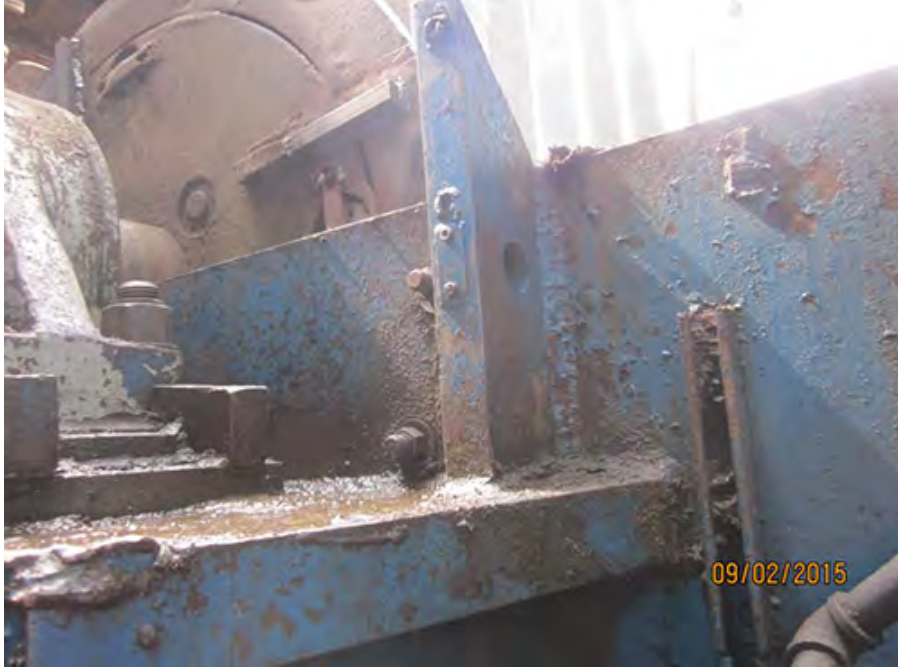
Bearing pedestals in good condition with no evidence of weld repair to the base
