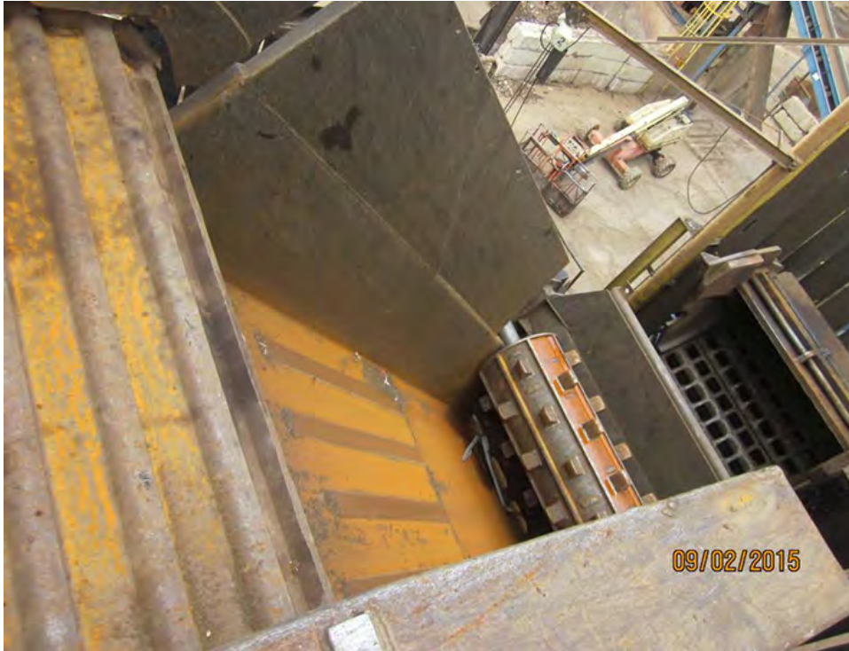
Main floor and side walls in excellent condition with new installed wear strips
