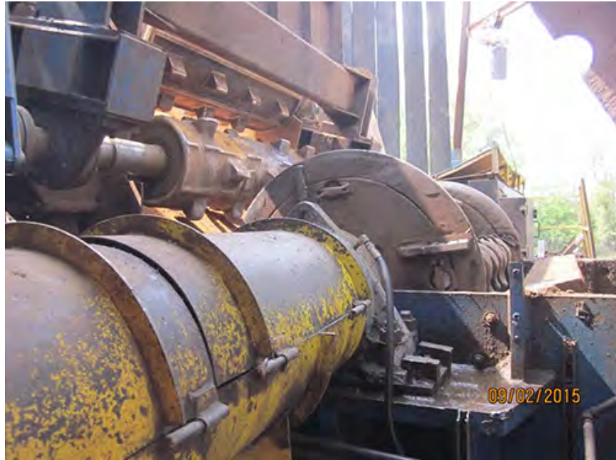
Safety cover excellent condition
