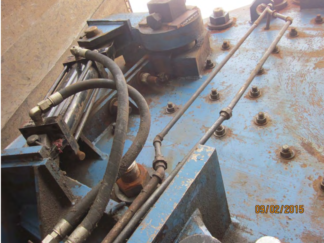
Reject door fabrications and reject door casting pivot attachment in excellent condition . No hydraulic leaks in cylinder
