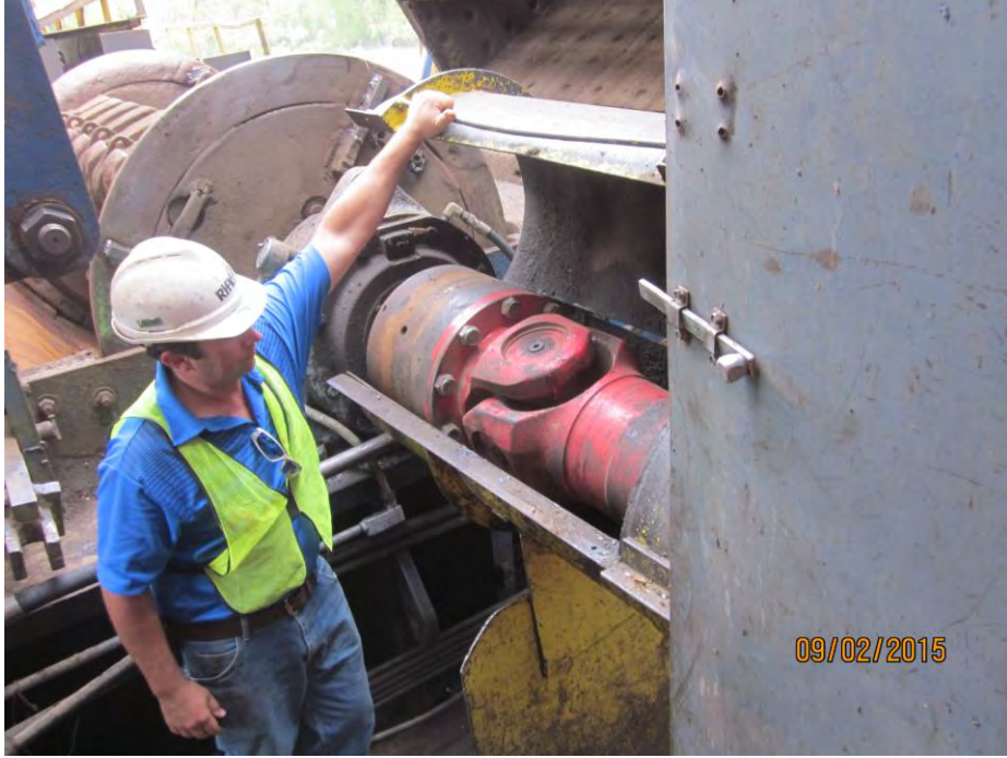
Rotor coupling to drive shaft in excellent condition
