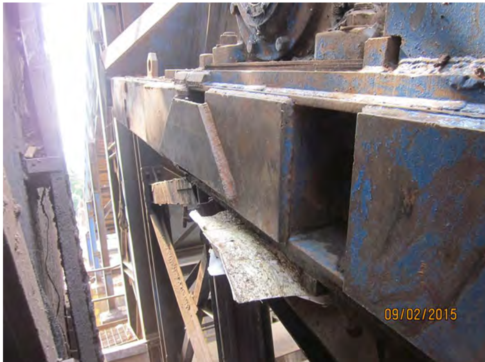
Feed roll frame in good condition straight with no evident weld cracking or twisting
