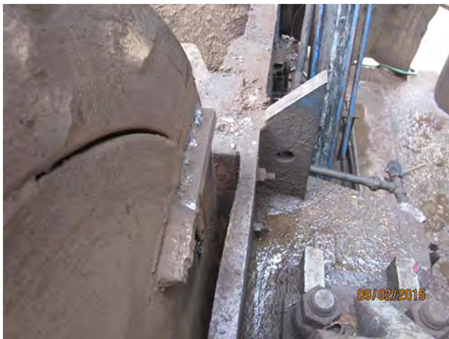
Small amount of wash on mill base side walls should be weld repaired. New wipers on rotor disc have been added that will help this condition.
