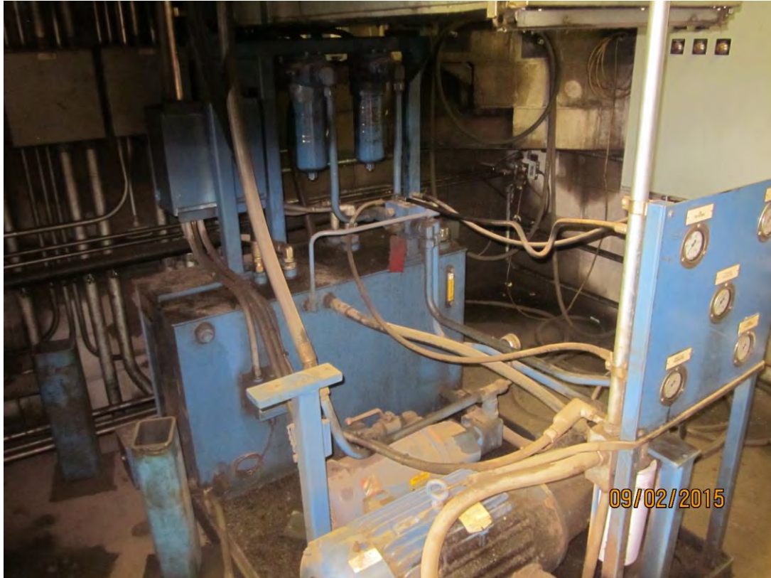
Feed roll drums and recirculating pump All hydraulic tanks in great condition free of hydraulic leaks and new filters installed All oil under pumps dry and clean
