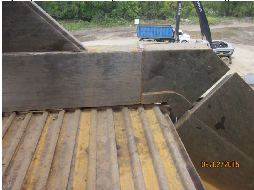
Transition from Infeed Conveyor to chute excellent condition. Side walls great condition.
