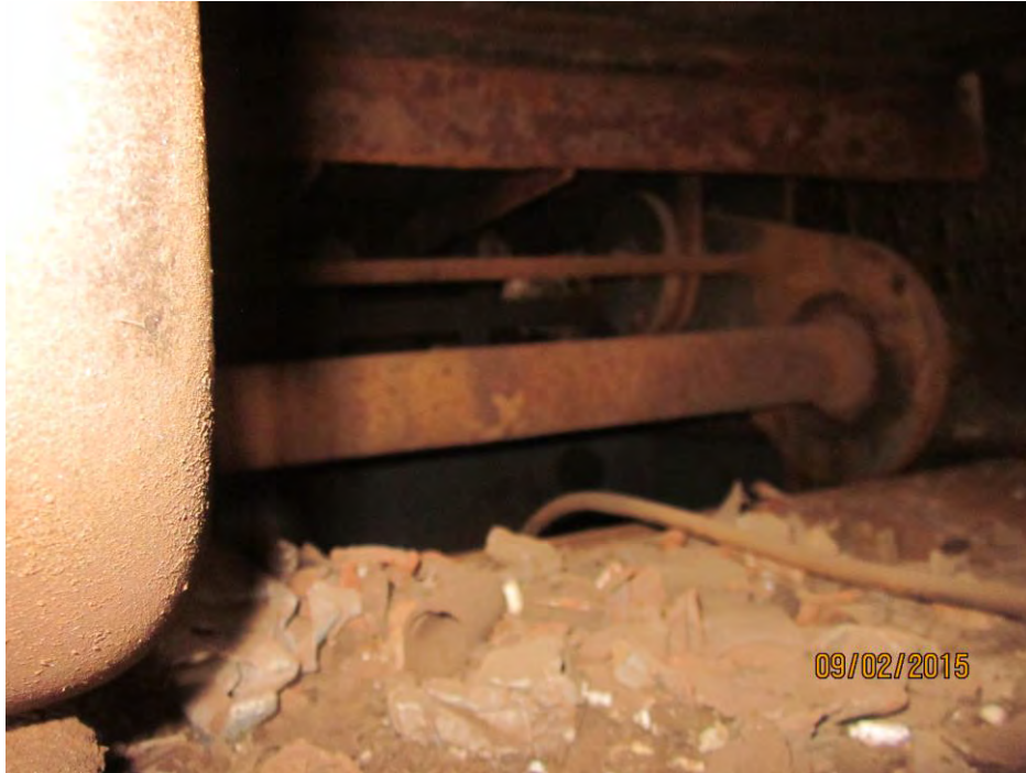
Considerable rust on eccentric drive shaft. Cover should be removed and greased
