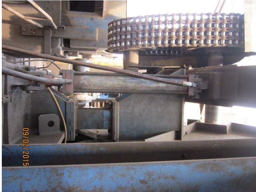
Feed roll drum chain drive, sprockets and chain in great condition. No hydraulic leaks from drive motor or feed roll hydraulic lift cylinder( Photo rotated 90 degrees)
