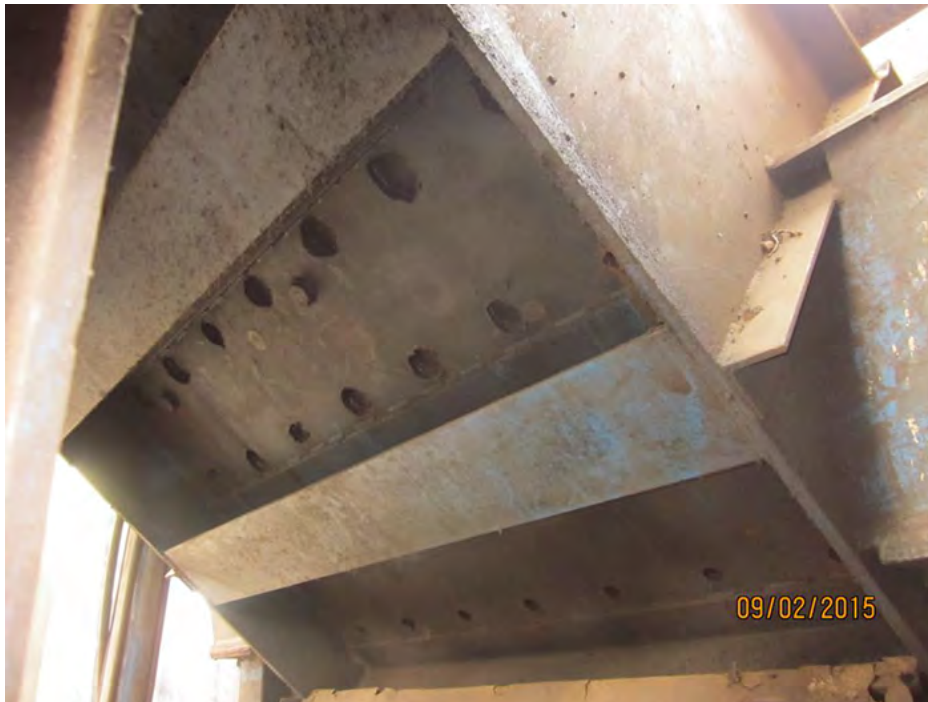
Plug welded floor liners seen under bottom of feed chute
