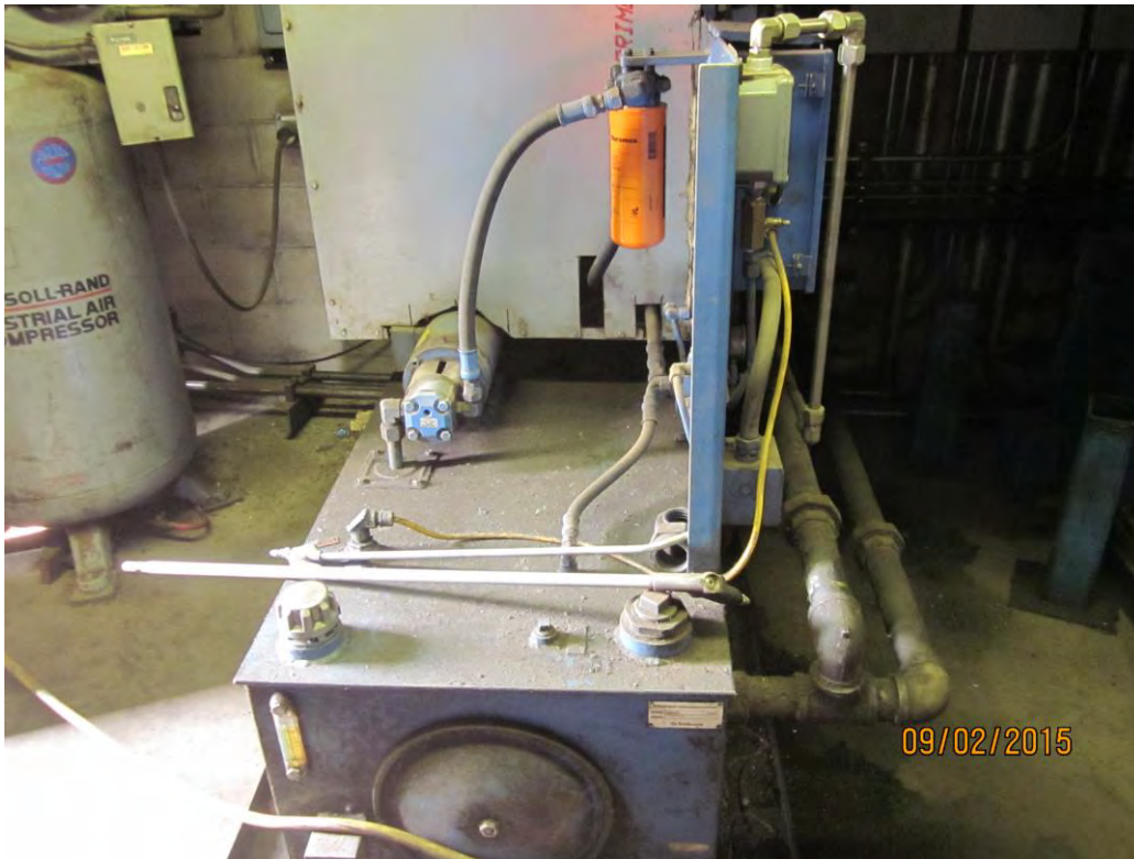
Bearing lube unit
