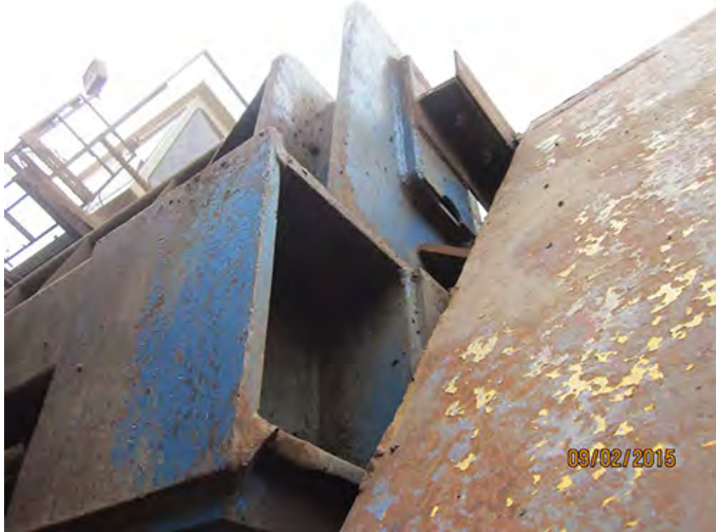
End of the feed roll frame boxed section all welds intact with no cracking
