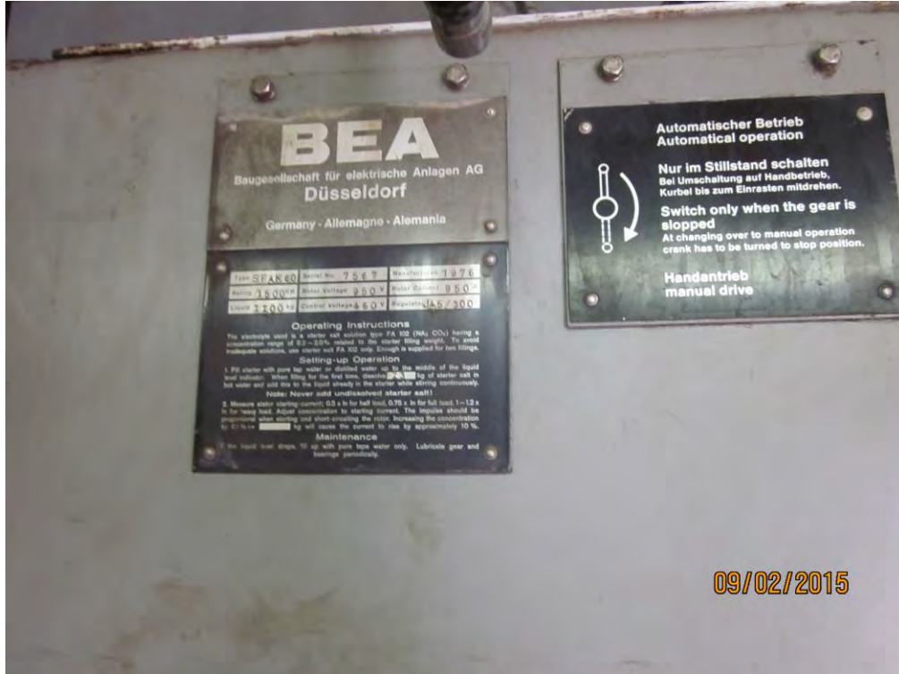
Motor Liquid Rheostat in good mechanical condition
