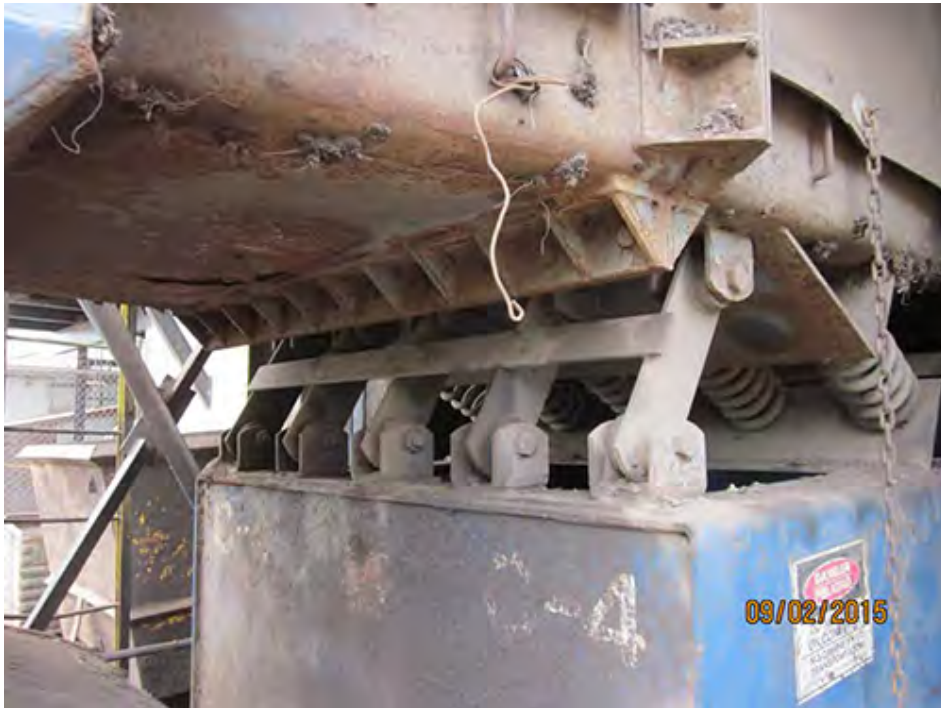
Exit trough pan has rust thru occurring
