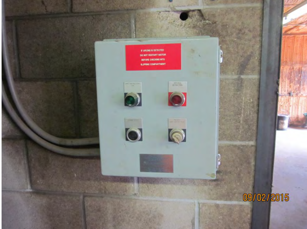
Motor Arcing detection
