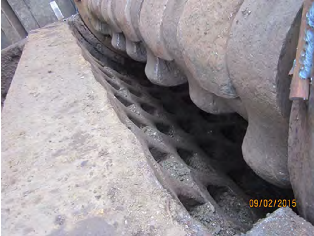
Double beam 4.25" x 8" openings staggered appear to be in good condition ½ life
