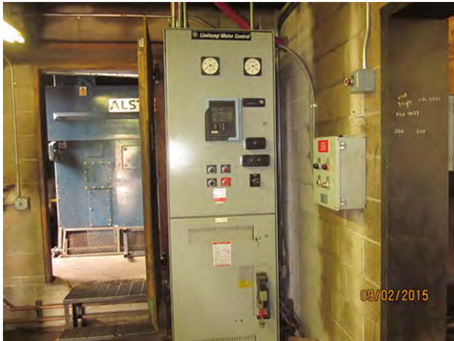
Main Motor control
