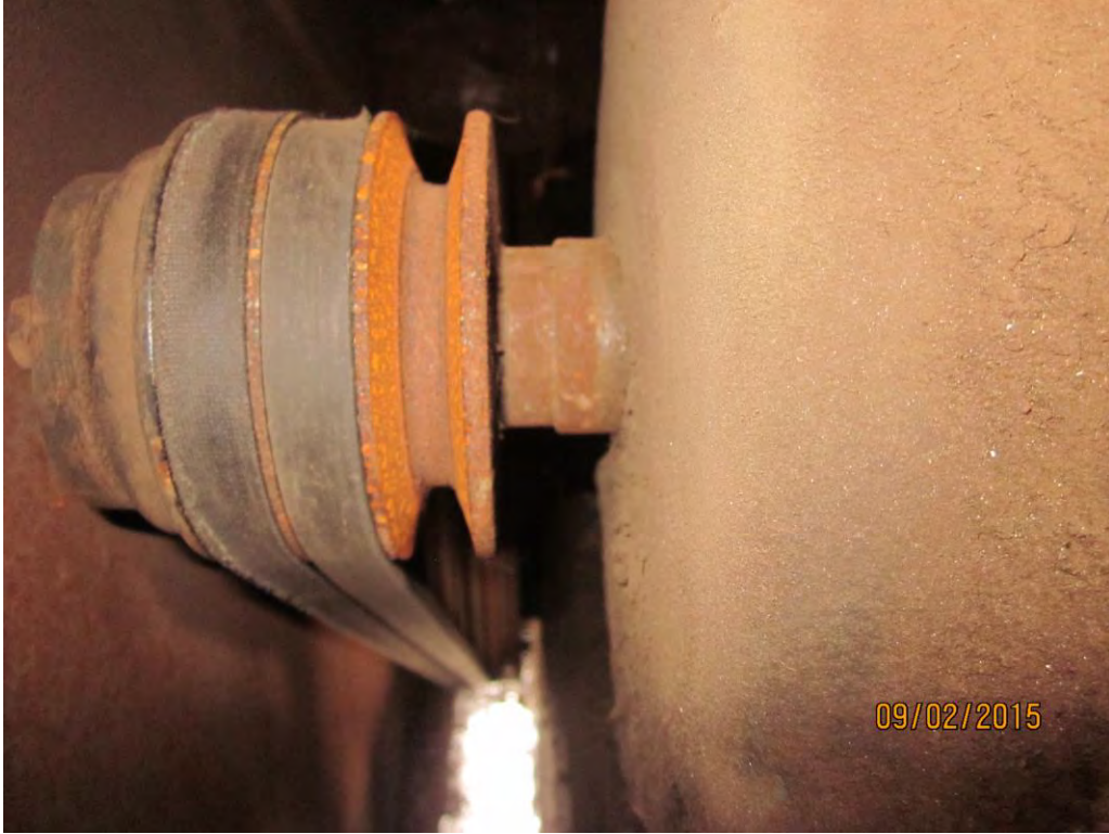
Pulley belt missing that drives the eccentric
