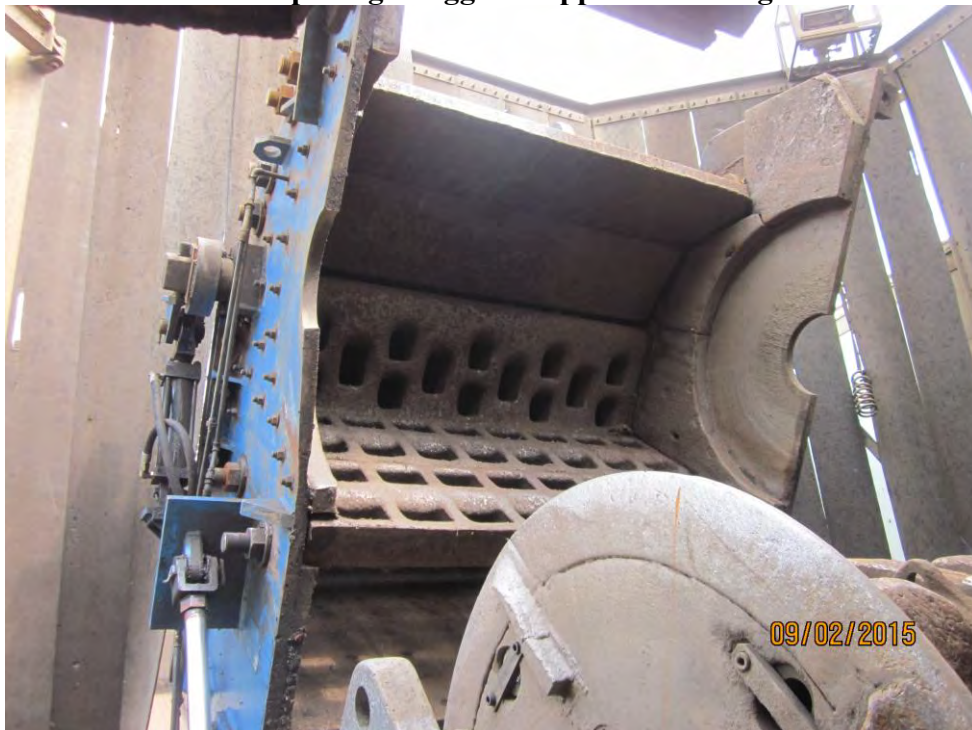
Reject door front wall liners and side wall liners appear in good condition. Minimal wash on side wall track facing rotor end discs.
