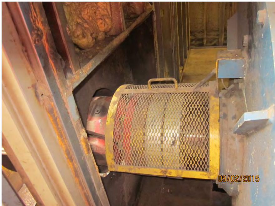
Motor coupling end with guard excellent condition
