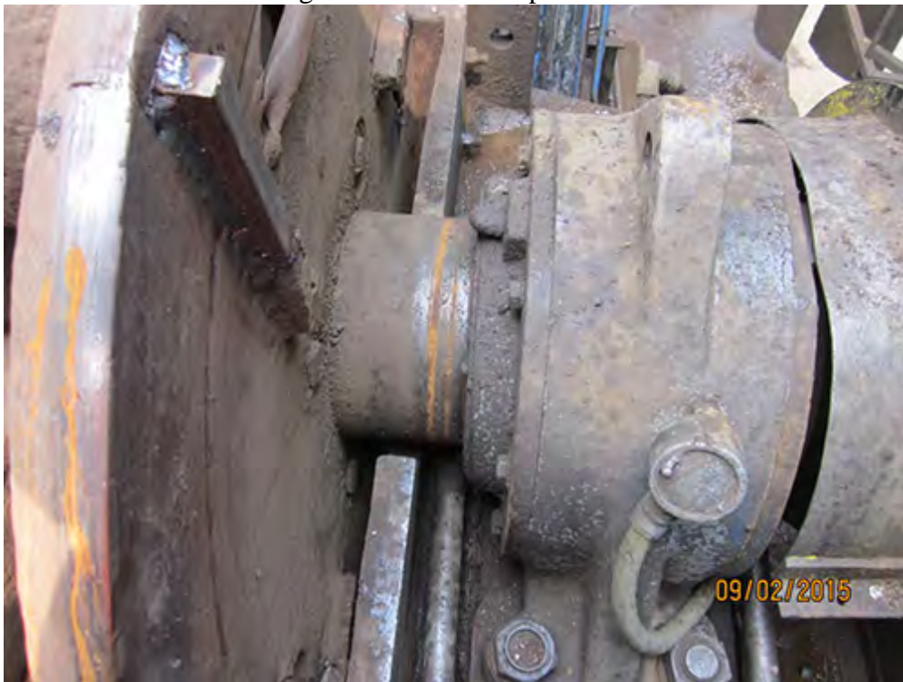
Bearing temperature probes in good condition both side. Minimal oil leaks from bearings.
