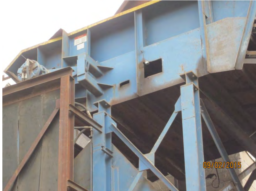
Hydraulic motor drive pulley clean and free of hydraulic leaks head shaft in good condition
