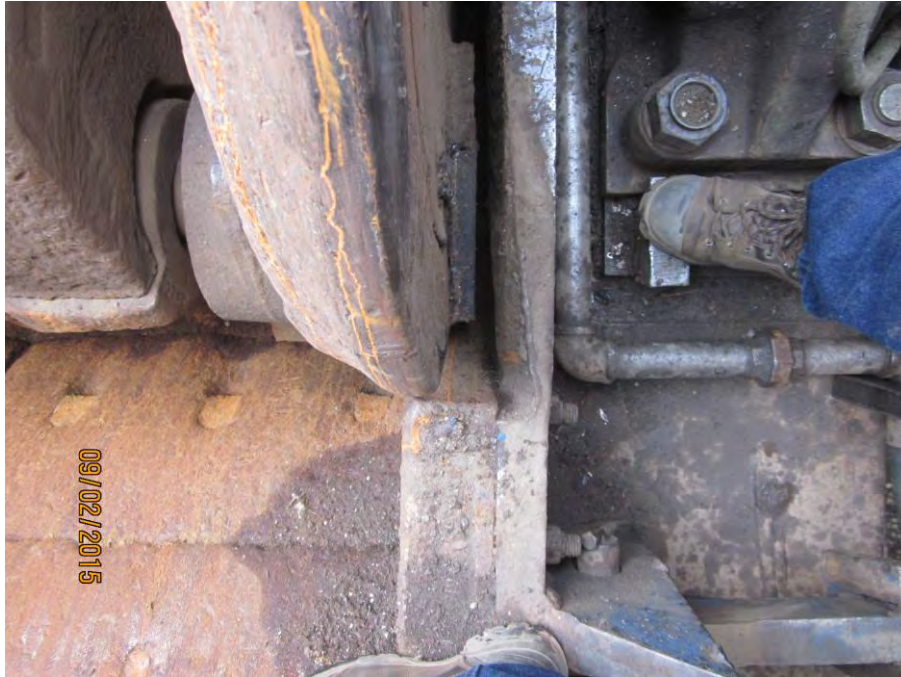
End discs caps need to be replaced extreme wash from the material impacting the end disc face. Side chute entrance liners should be replace and for additional protection.
