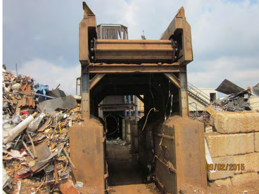
Tail shaft pulley and tail shaft pillow block bearing in good condition
